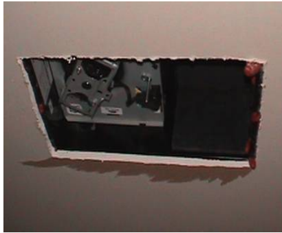
Figure 43 Paper tear in ceiling panel
