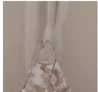
Figure 41 Mud lump in bottom of corner
