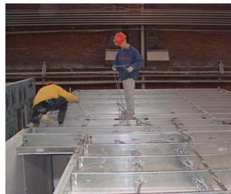
Figure 23 Wiring on top of a module
