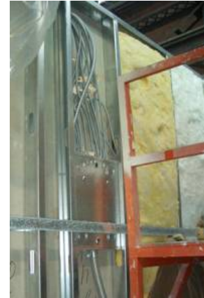
Figure 50 Insulation void at electrical panel
