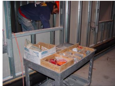
Figure 28 An electrician's cart
