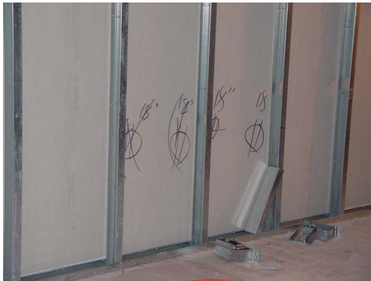
Figure 8. Incorrect location markings for electrical boxes
