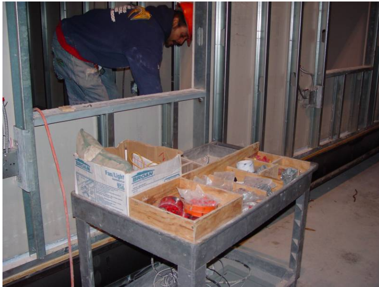
Figure 12. Electrical supply cart staged outside module
