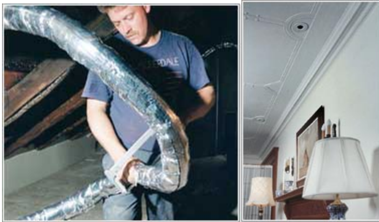
Figure 3.8 High velocity duct (left) and finished installation (right) (Spacepak)
