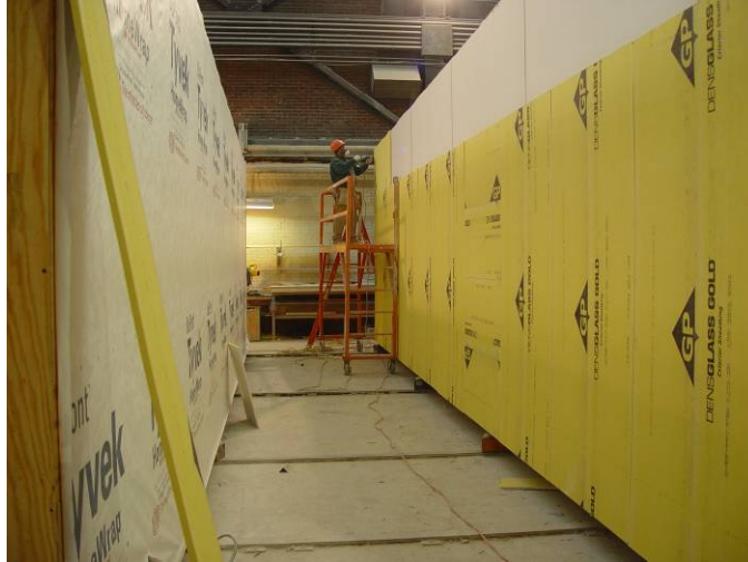
Figure 20. Additional installation required for yellow drywall
